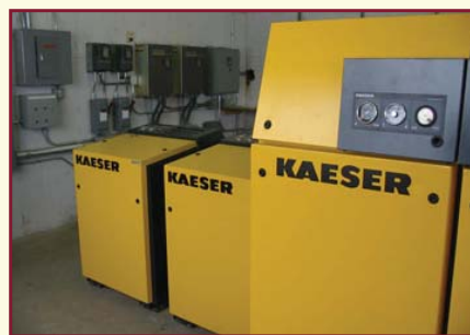
The goal was to use four rotary blowers to upgrade from the existing gravity-fed system to a controlled pressurized distribution system.
