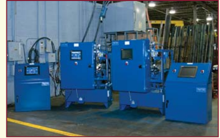
Sorensen Systems designed and built three hydraulic power units and a PLC driven control system to remotely operate the gates from the passenger embarkation station on the San Antonio River Walk tourist attraction.
