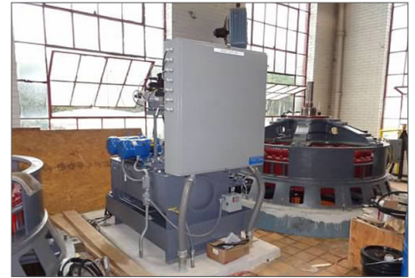
Sorensen Systems designed and built turbine control panels and balance of plant control panels as part of the Spartanburg Water Treatment improvement project.
