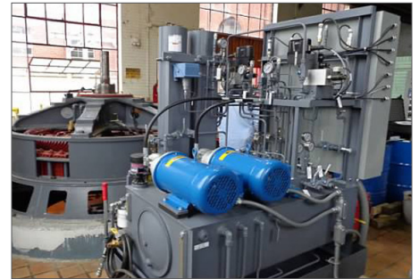
The Spartanburg Water Treatment plant operates two 500 kW turbine generators providing water treatment and power generation to 200,000 consumers including neighboring counties.
