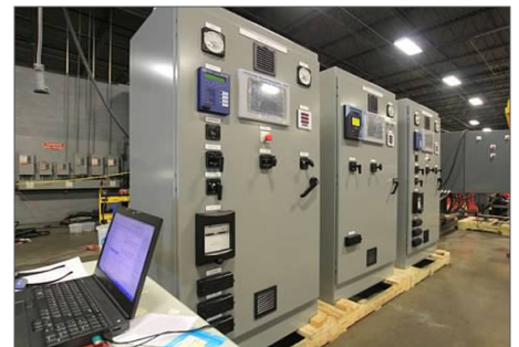
The refurbishment included new PLC based unit control systems, one per generator, which were programmed and tested at the Sorensen Systems fabrication facility.
