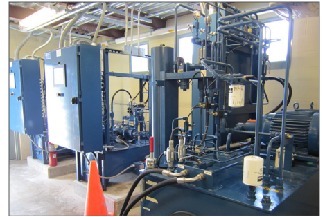
A control system was required for the setting and monitoring of water levels and new locks for the famous San Antonio River Walk excursion boat tourist attraction. This involved design, construction and start-up of three power units and two remote operator panels for controlling the lock system.
