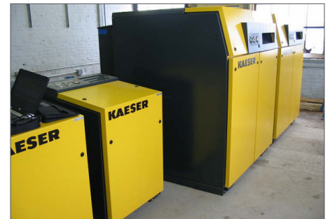
The four low pressure blowers installed at NH Gas in Keene NH were designed to cover a wide cfm range and to serve as internal back-up during routine maintenance.
