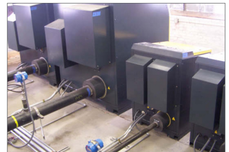
The ambient air, gravity-fed system needed a boost from the low-pressure blowers as demand for propane gas increased from residential and commercial expansion.
