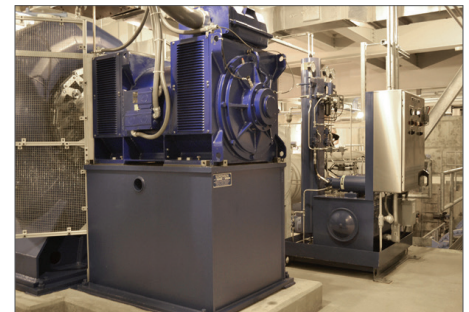
The 200 kW, 480 VAC, 3PH, 60 Hz, 727 rpm induction generator was manufactured by Marelli Motori.
